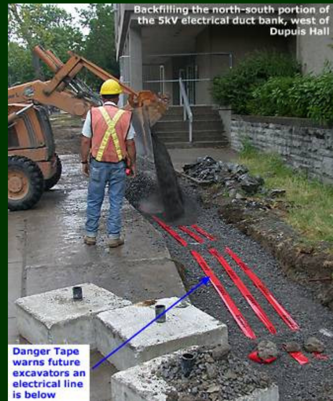
“Chairs” maintain spacing between electrical ducts.
