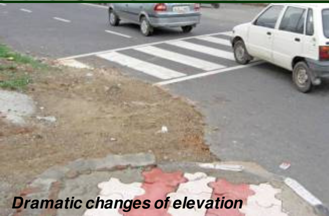
Uneven pavement surface due to lack of proper setting in a concrete sub-base.
