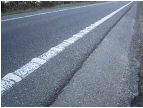
Figure A.11: Example of longitudinal ATLM (Source: Secretariat CAREC 2018. CAREC Road Safety Engineering Manual 2: Safer Road Works)
