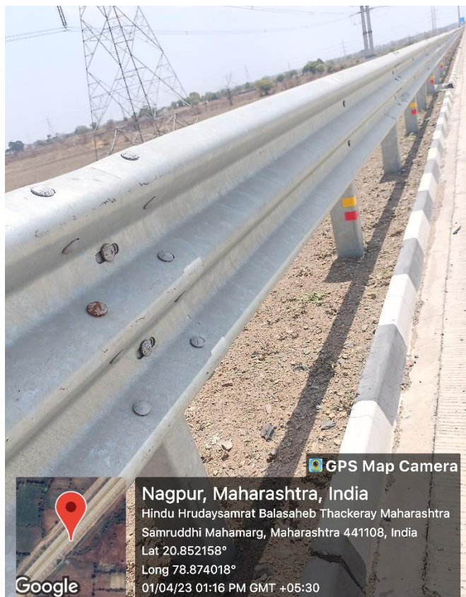
Figure 4: Semi Rigid Crash Barriers Provided to Entire Expressway
