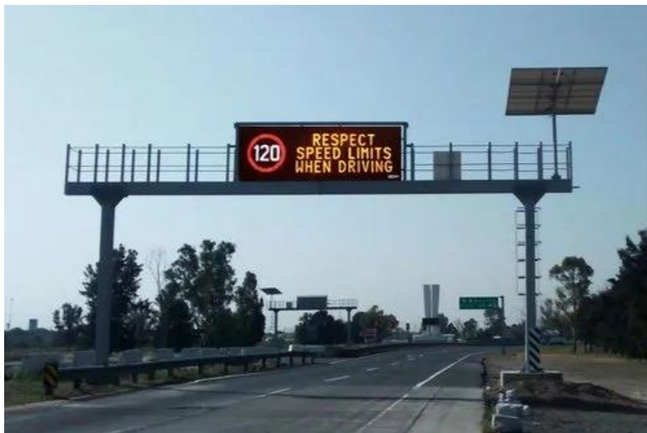
Figure 43: Variable Sign Board
