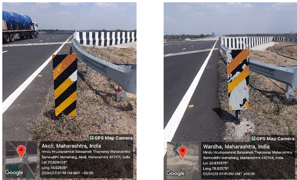
Figure 58: Worn out hazard markers were observed during road inventory survey
